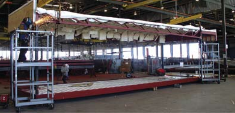
The building sections are manufactured in a factory-controlled setting while the building's site is simultaneously prepared.
