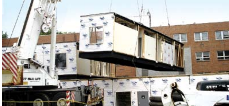
The modules are shipped to the site and set upon the already prepared foundation with the use of a crane.
